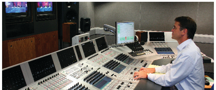
The new 72-fader Vista 8 Installed in BBC TC6
